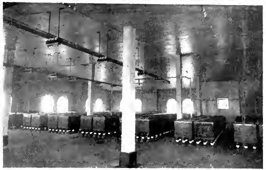
FIG. 4.—GENERAL VIEW OF STORAGE BATTERY ROOM
